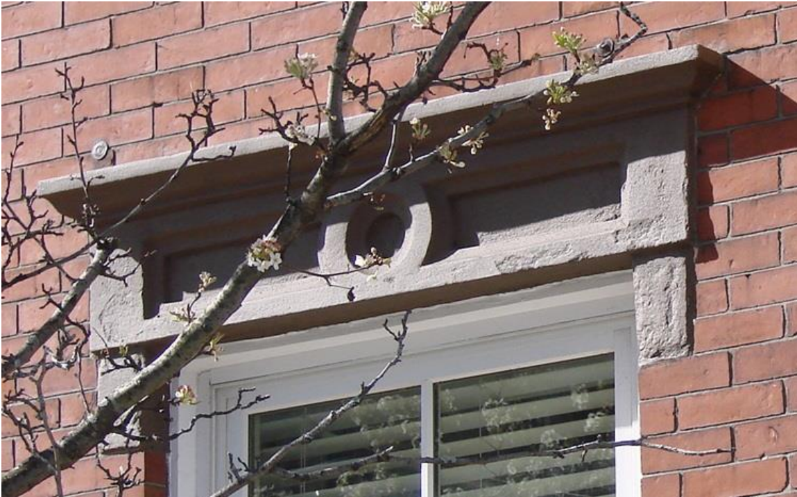
72 High Street first floor lintel detail
